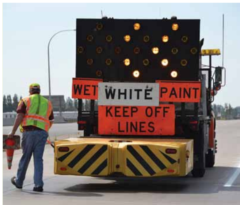
AFSCME’s striping crews in MnDOT dispel the myth that the private sector is more efficient than public employees. The AFSCME crews in Minnesota paint lines on highways for half the price that private competitors charge.
